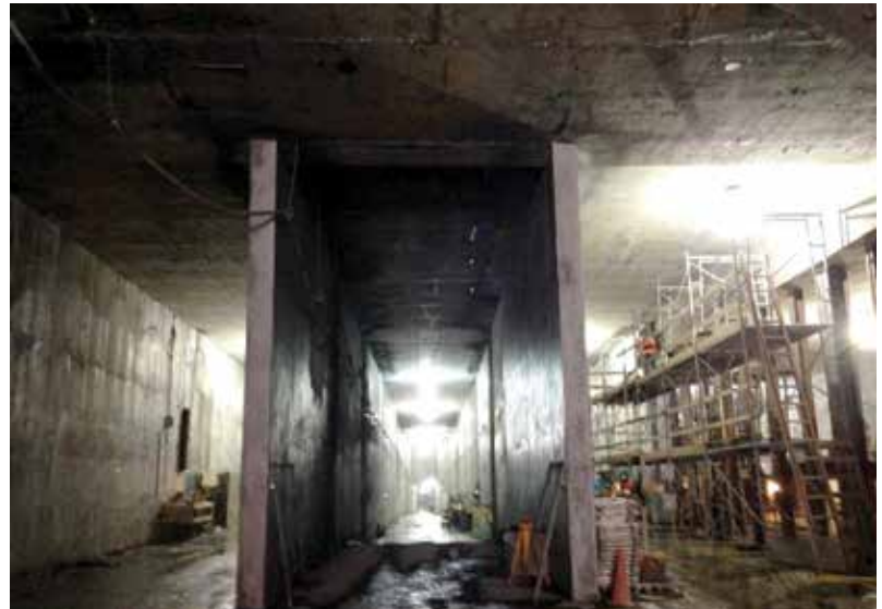
Fig. 4: Each of the three bays shown is a future train corridor for Long Island Railroad. To the right you can see square columns
