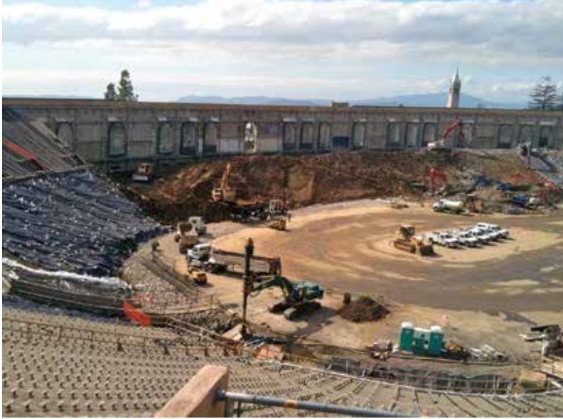
Fig. 1: Overview of the existing historic walls during demolition and excavation. A layer of shotcrete was later applied over the existing walls in various thicknesses from 5 to 36 in. (127 to 914 mm)
