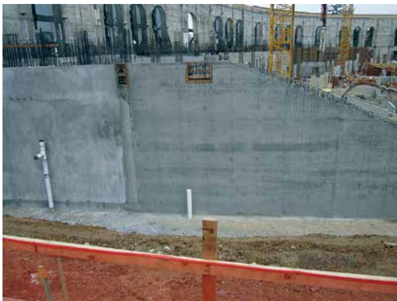
Fig. 7: Shotcrete shear wall after the forms were stripped. The right side of the wall is the stripped form side. The left side is the shotcrete steel trowel finish side
