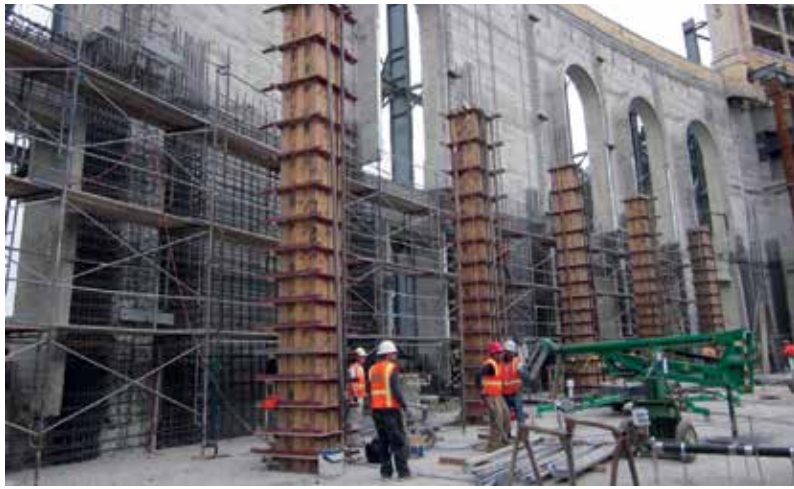
Fig. 5: Application of 40 ft (12.2 m) tall shotcrete layer 36 in. (914 mm) thick over the existing historic perimeter wall
