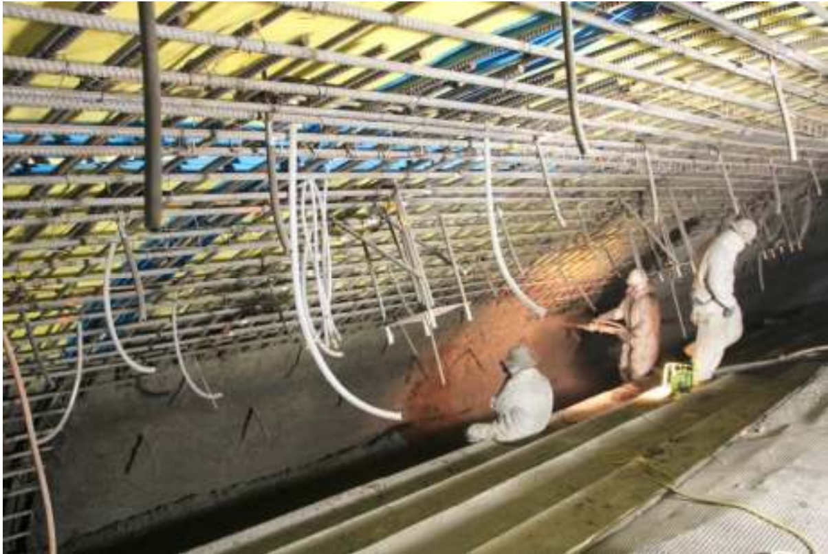
Arch lower panel being built up, not the BA anchors and hoses running out displaying what the full depth is
