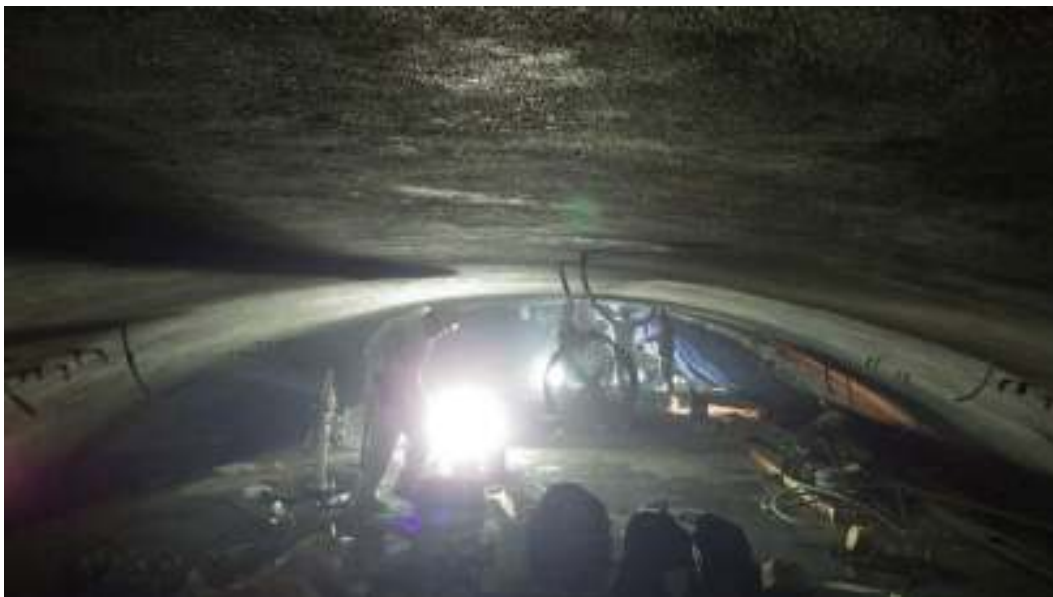
Working the final panel, ventilation needed and made curing a challenge as the heat was a challenge to manage on a daily basis.
